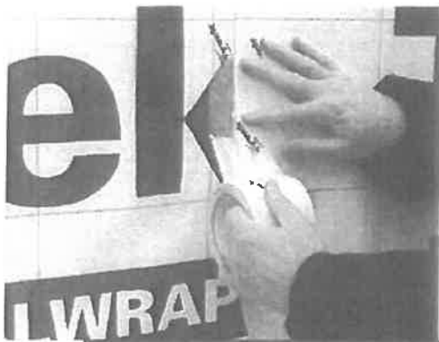
Taping the seams after wrapping is the best practice for completely sealing the building envelope.
